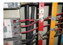
Outer insulation damaged in live electrical wires
