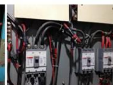
Properly Maintained MCC Panel - Ideal Case
