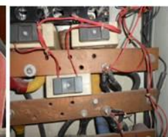
Unsafe method of connections from joints without using proper lugs
